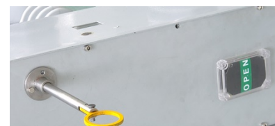
Lockout handle-pulled (open position)
