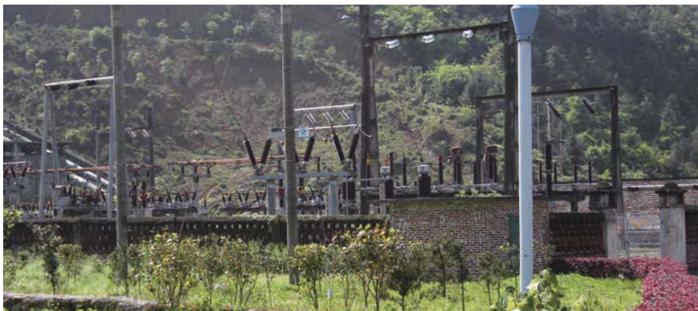
220kV Surge Arrester - China Grid installation – 2005
