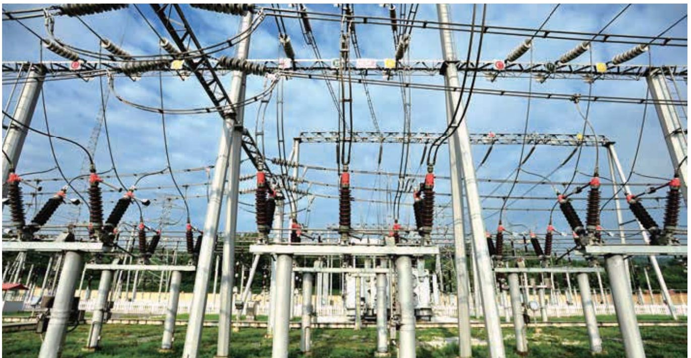
110kV Surge Arrester - South Grid installation – 2002
